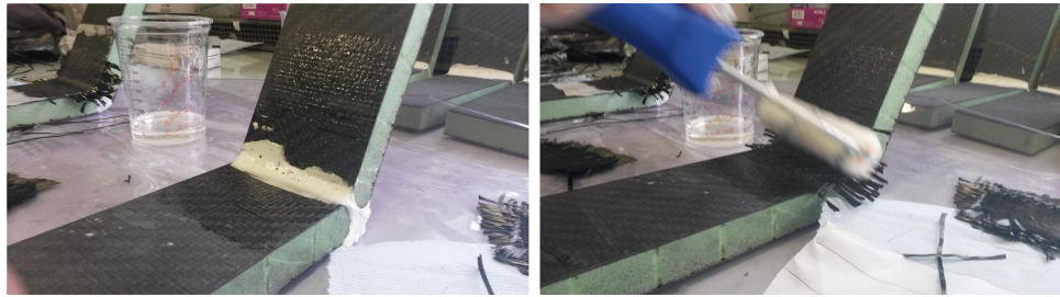
Figure 76: The inner joint carbon fibre reinforcement made using wet layup of four carbon fibre plies.
